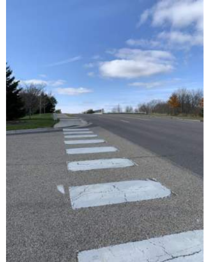
Picture 6 – Looking West (Stopped Beyond Stop Bar)
